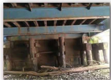
The 63-year-old creosote timbers are rotting.
