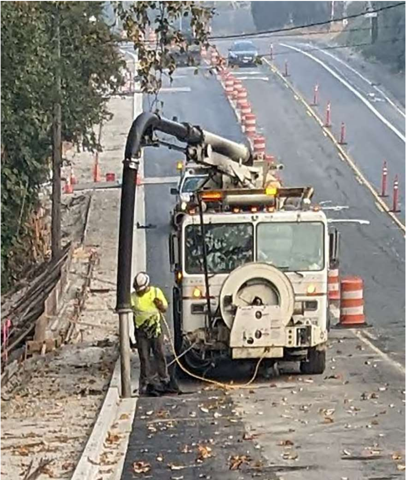
Oct. 19, 2022 – It takes a massive hose to suck up any construction debris to clean the freshly poured gutter and curb. This makes sure the new drainage system is ready for wet weather.
