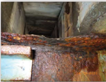
We are losing sections of steel.
