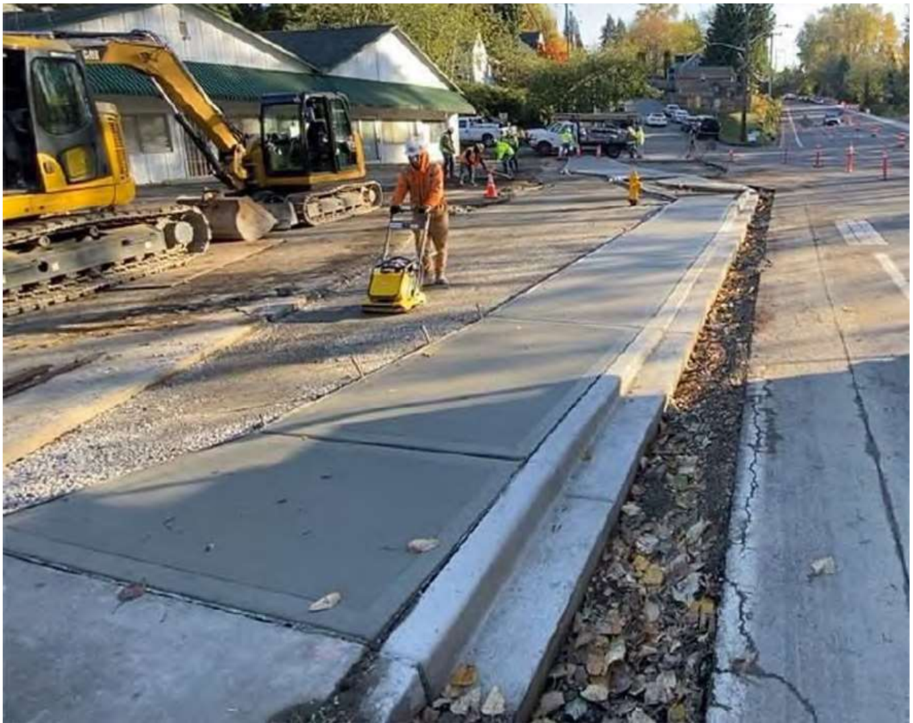
Nov. 14, 2022 – Multiple crew members clean and clear the driveway near S 116th Place and Renton Avenue S before it is paved.
