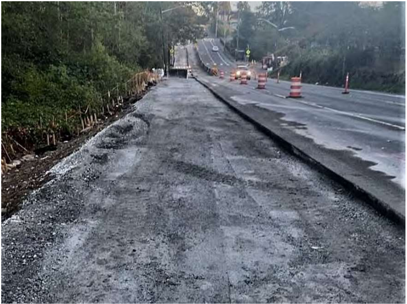
Sept. 29, 2022 – Crews prepare the westside shoulder of Renton Ave. S for a new curb, gutter, and sidewalk.
