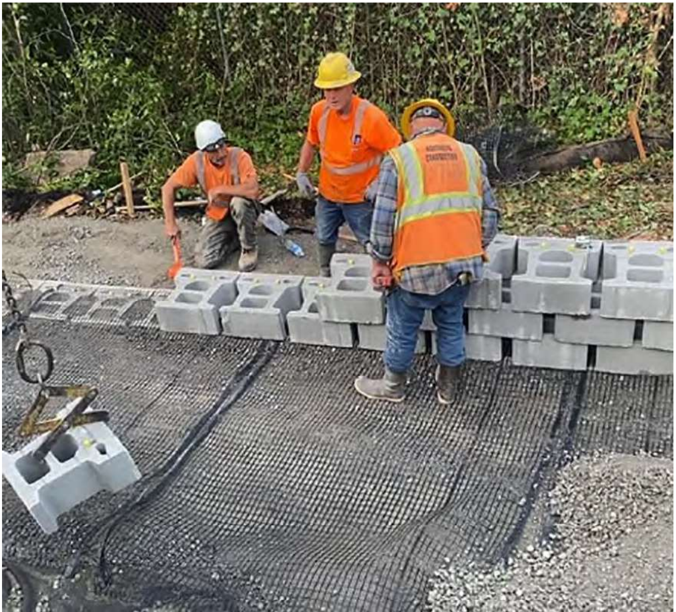
Oct. 5, 2022 – Crew members build a supportive wall for the sidewalk which will go down Renton Avenue S.
