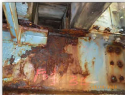
The super-structure is 108 years old and severely rusting.
