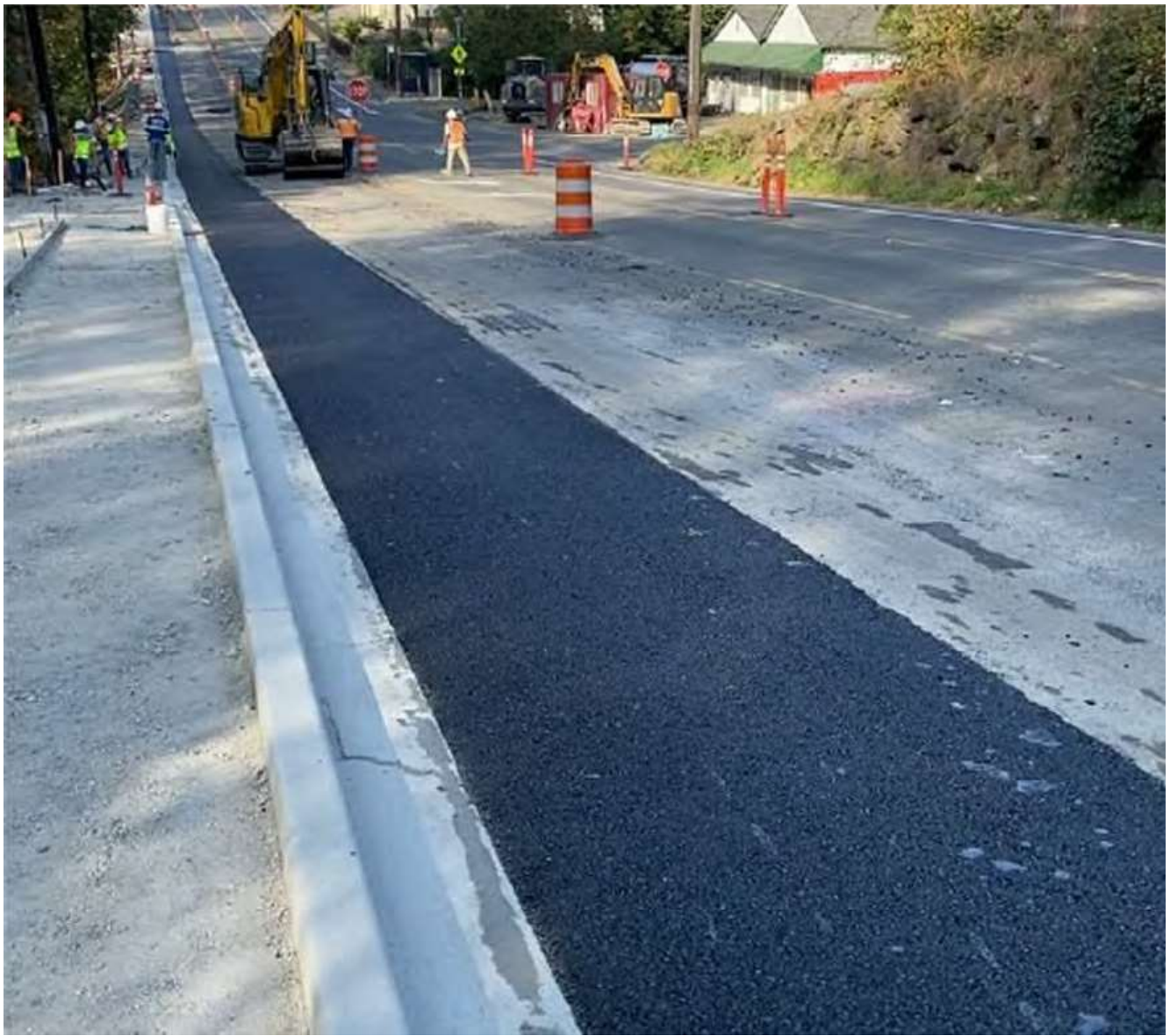
Oct. 17, 2022 – The finished curb continues north down Renton Ave S. The bike lane and sidewalk come next.
