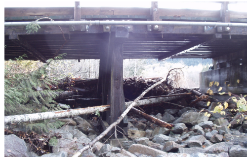
Figure 7: approach span and debris jam – looking upstream
