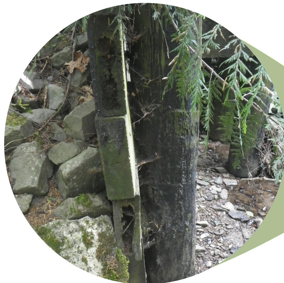
Decaying timber support structure
