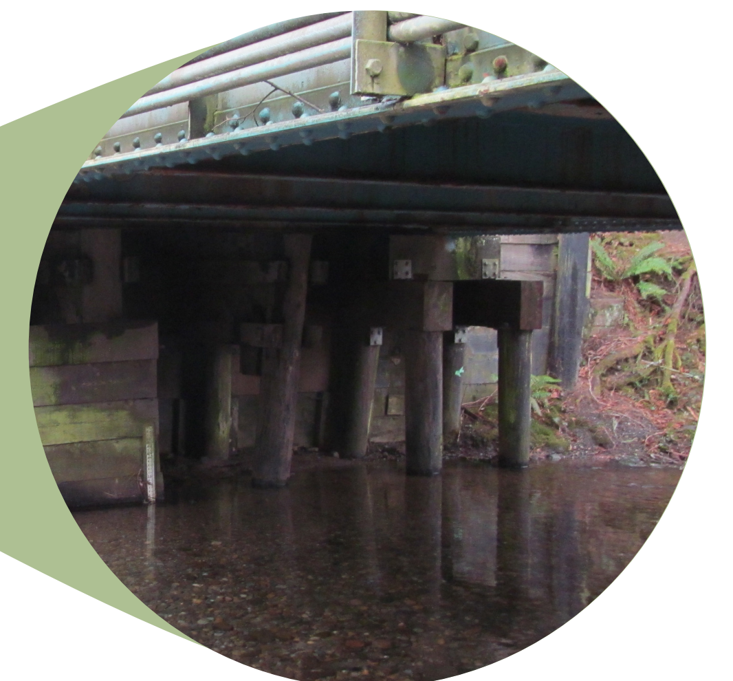
Creosote-treated timber piles in environmentally sensitive creek
