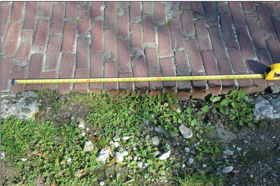
Figure 11. Missing edge restraint segment.
