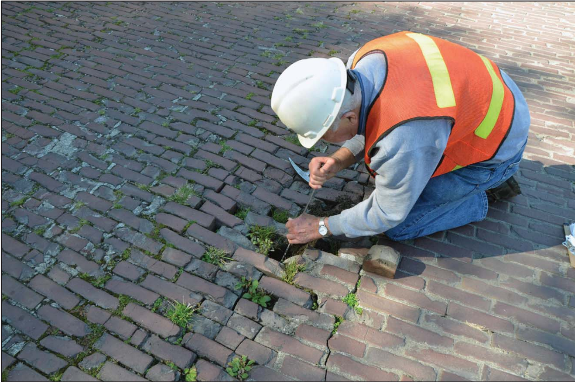
Figure 10. Test probe 46 with loose brick.
