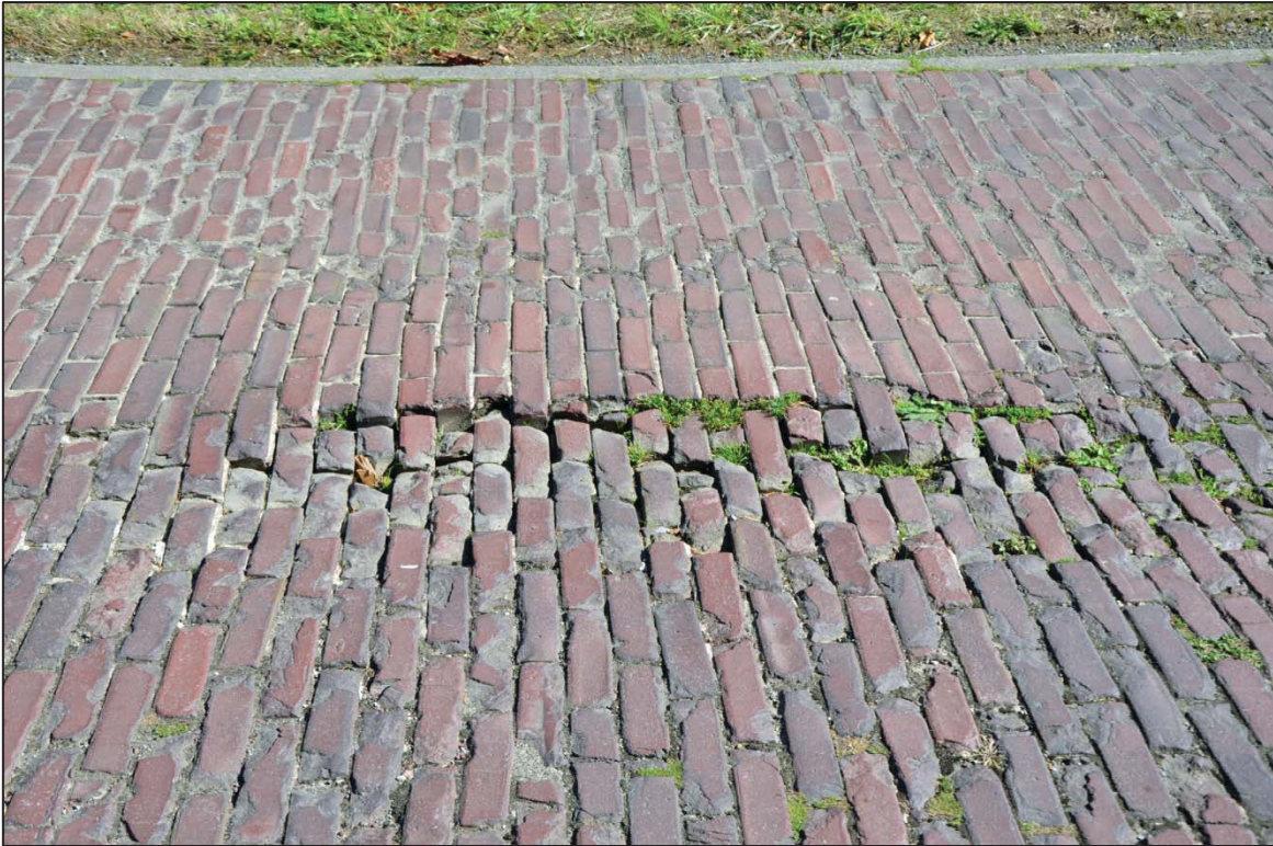
Figure 12. Road segment with fractured brick.
