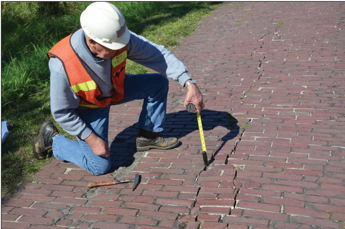
Figure 9. Test probe showing failure of sub-base.
