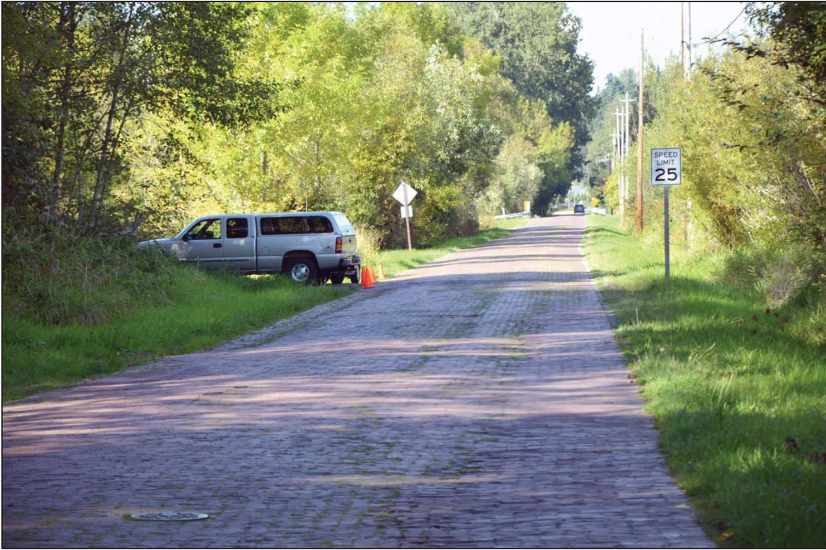
Figure 8. Surface settlement showing apparent subgrade bearing failure (note sag in road on left side of photograph).
