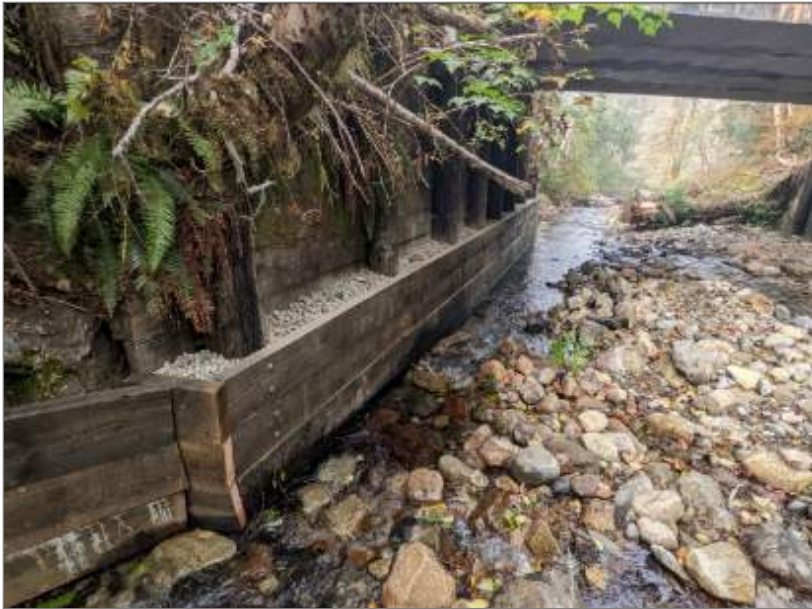
Granite Creek Bridge No. 359A – Fender wall added to protect the abutment backwall from scour
