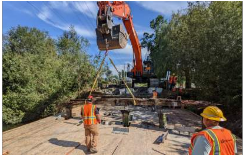
Newaukum Creek Bridge No. 3063 – Removing decayed timber caps from a work platform
