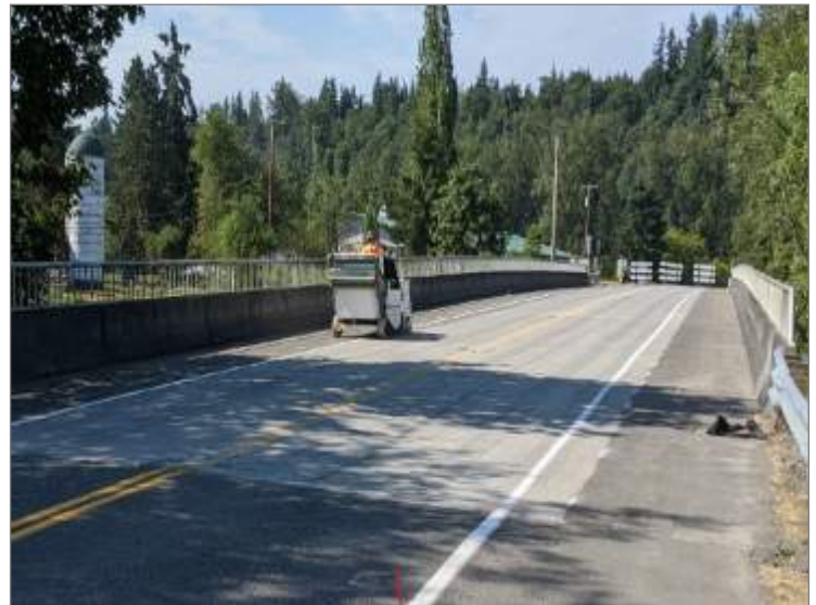
Whitney Bridge No. 3025 – Shotblaster preparing the deck for application of epoxy overlay
