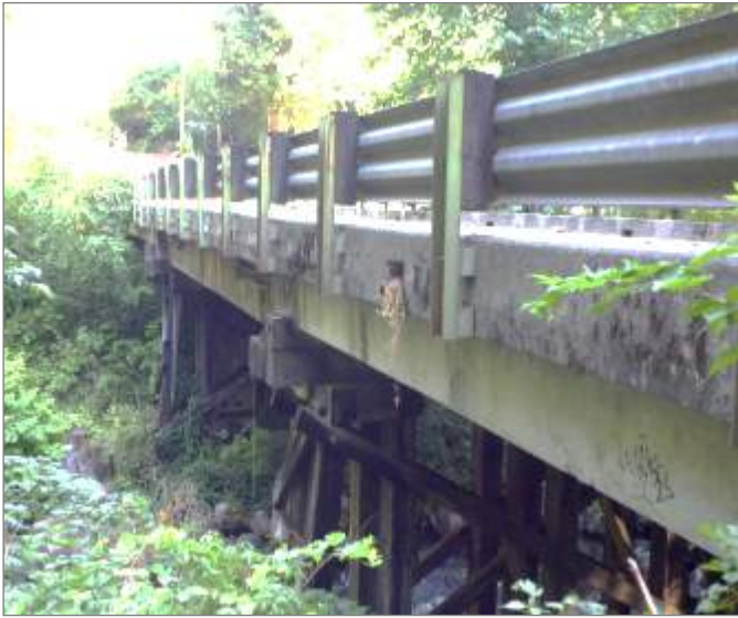
Upper Tokul Creek Bridge No. 271B – Timber substructure supporting concrete deck units
