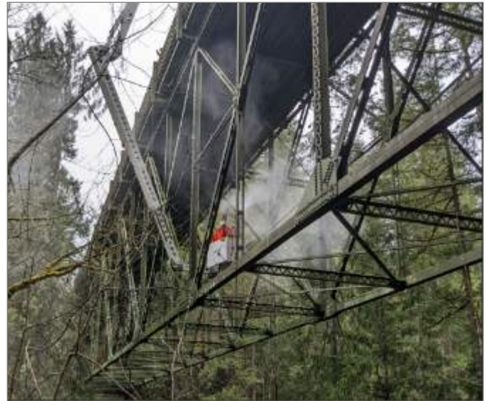
Washing lower truss members of the Green River Gorge Bridge No. 3032 in January 2023
