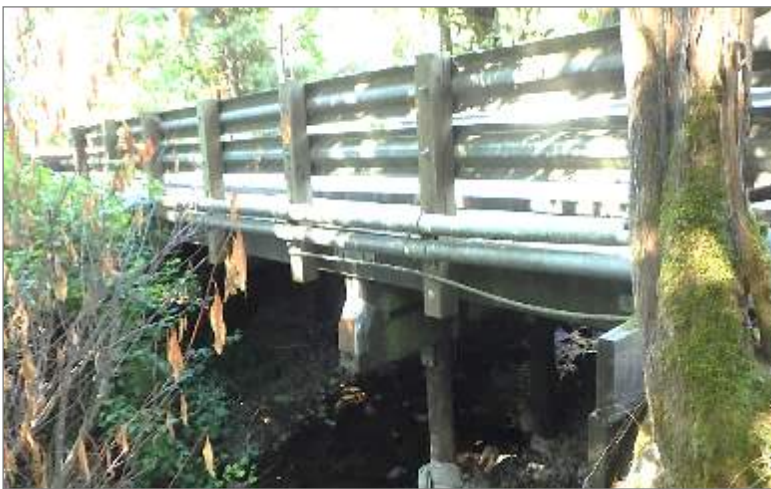
Fifteen Mile Creek Bridge No. 493C – South elevation of timber substructure and stringers
