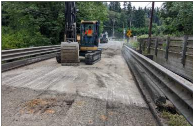
Covington Creek Bridge No. 3085 – Removing asphalt surface down to the concrete slab
