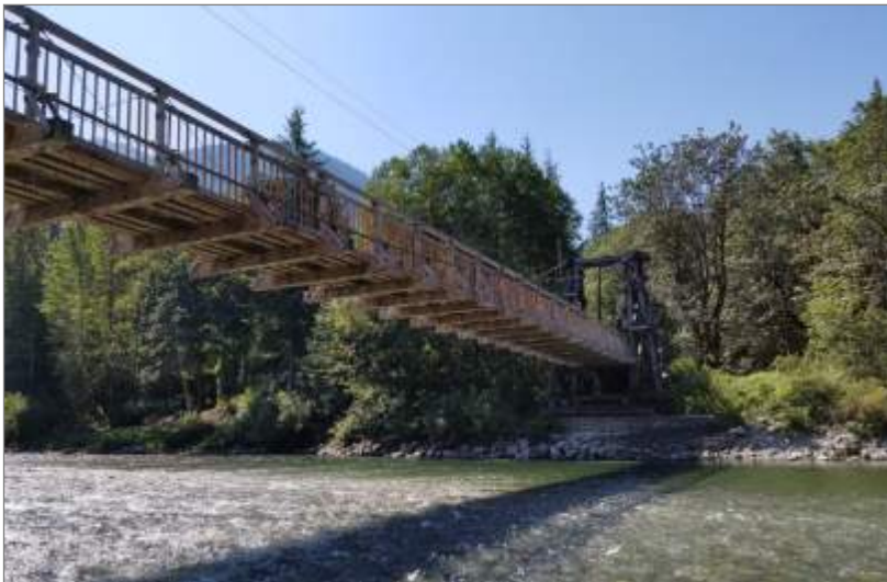
Baring Bridge No. 509A – South tower and timber truss of suspension bridge spanning the Skykomish River
