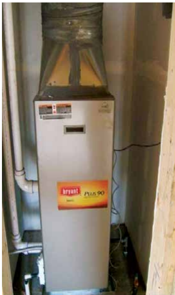
High Efficiency Energy Star Furnace with direct vent and condensate line. This furnace also includes ducted fresh air (not shown in the photo). Source: O'Brien & Company.
