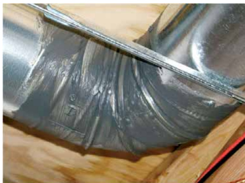
This metal duct elbow seam is properly sealed with duct mastic. If the ducts are in the crawl space, attic, or garage, they should be insulated after being well sealed. Source: O'Brien & Company.
