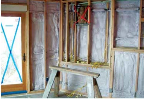
This picture shows the “flash” portion of a “flash and batt” installation. The flash coat of spray-in-place foam insulation creates a tight air seal. Source: O'Brien & Company
