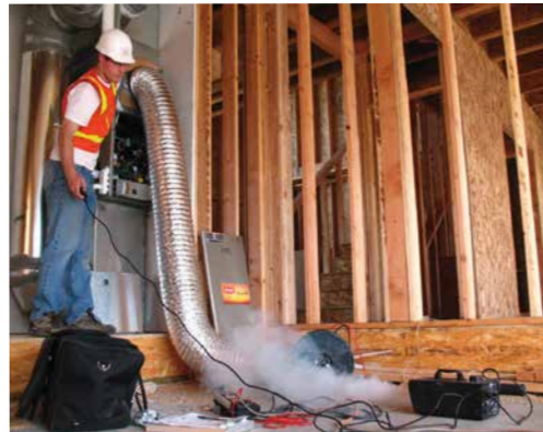
Duct leakage testing in a new home. Non-toxic smoke can be used to locate leakage areas, especially during framing in new construction. Source: O'Brien & Company.
