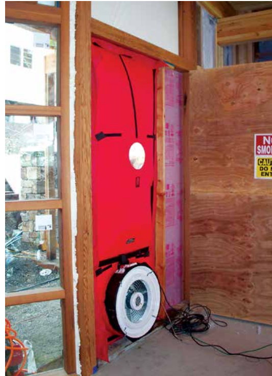
A blower door test during construction measures the home's air leakage at a standardized pressure. Source: O'Brien & Company
