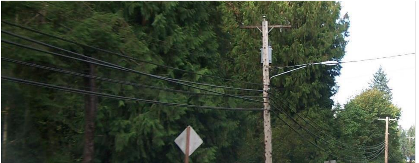
Figure 31: Utility Pole Requiring Make-Ready
