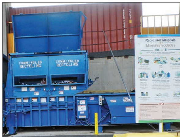
Compactors for recyclable materials
